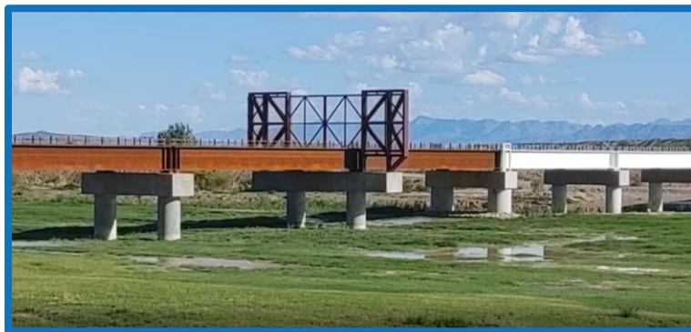
Presidio-Ojinaga International Rail Bridge in October 2019 – Scheduled for freight operation in April 2021 Credit: Brad Newton, Presidio Municipal Development District (PMDD)
