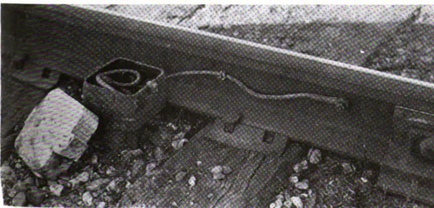
Pot-head arrangement for terminating Okosheath conductor, with Raco fittings
